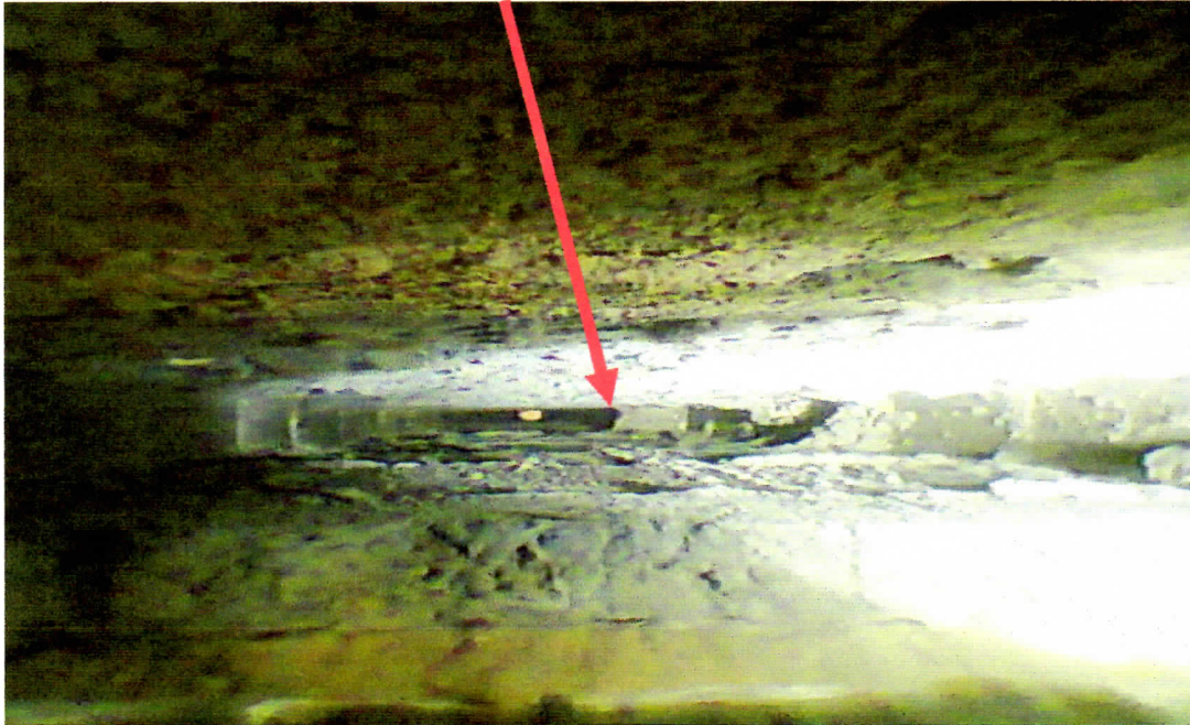
Photo of where the flue gases enter the wall, note the discolouration of the plaster wall.
